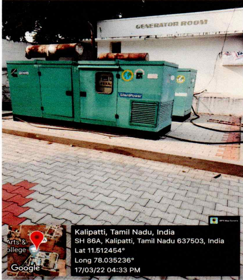
GENERATOR FOR POWER BACKUP
